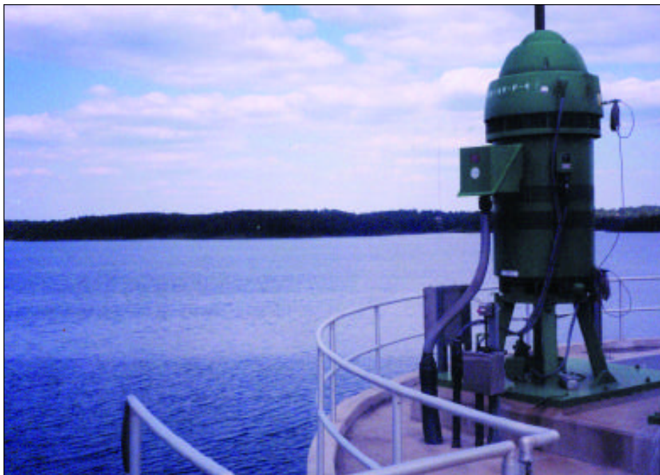
A high capacity pump withdraws raw water from the MWA Javors J. Lucas Lake (Town Creek Reservoir) for eventual drinking water production at the Amerson Water Treatment Facility.
