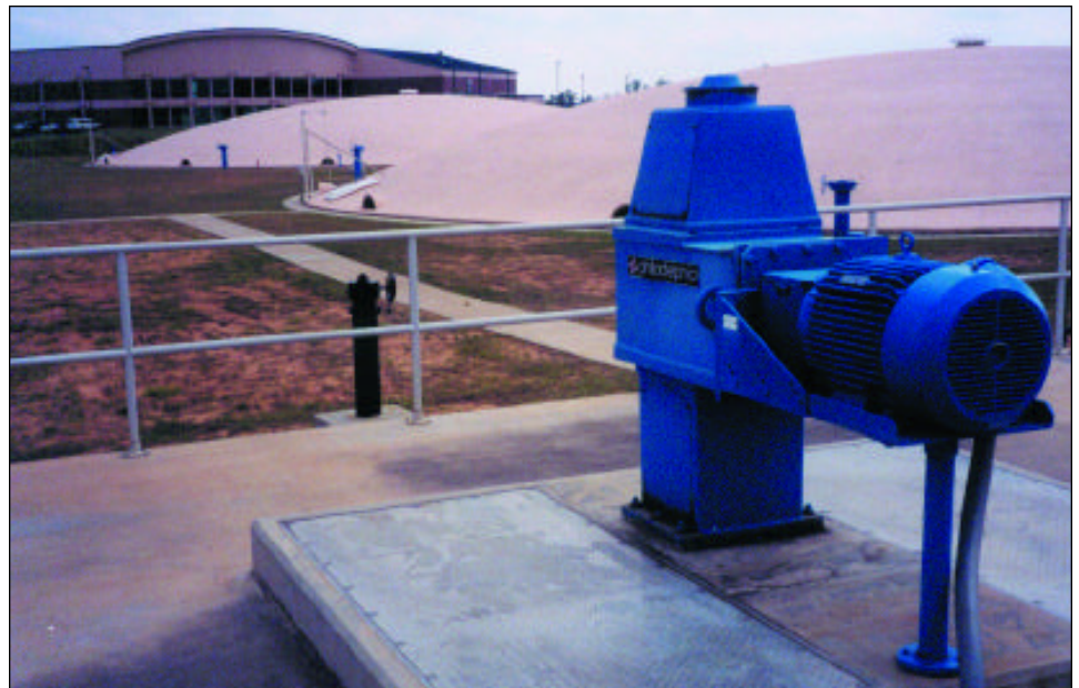
(Above) The new Frank C. Amerson, Jr. (Town Creek) Water Treatment Facility features the Macon Water Authority's (MWA) water production operations and water quality lab (building in the background), as well as clearwells (domes in the center) for storing finished drinking water that's pumped to MWA customers.
